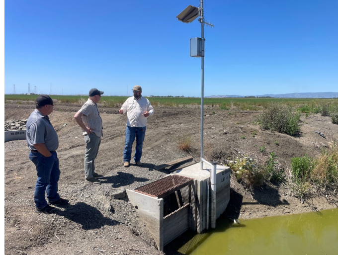
RD 2068 Lateral 4/5 transducer site
