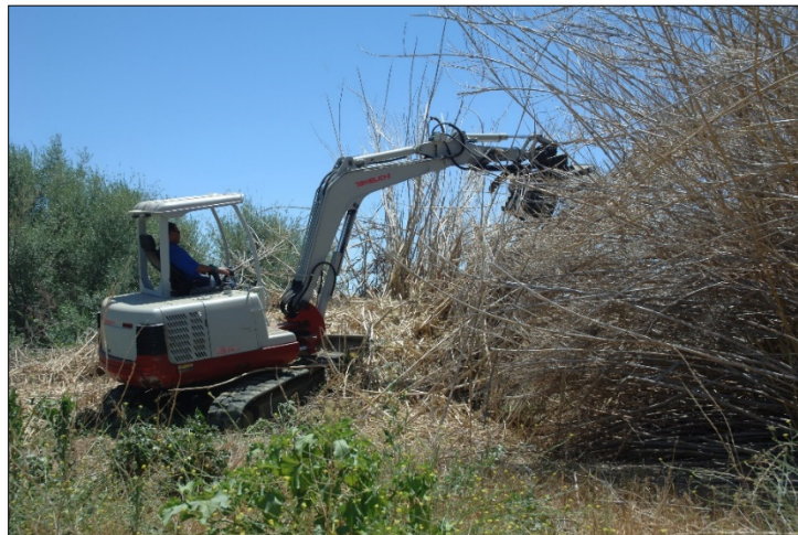
Mechanical (backhoe) removal of giant reed (Arundo donax) near the Cache Slough Complex region in northern California. Photo Credit: California Department of Water Resources.
